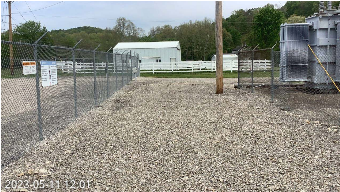
Photograph Location 3. Representative view of graveled substation within the Project area. Photograph taken facing north.
